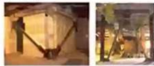
Figure 6. Friction dampers installed as diagonal and chevron bracing [10].
